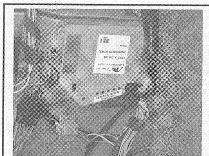
Fig. 72 This is the ABS module. It is located in the luggage compartment, mounted against the rear seat supports
