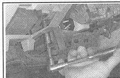
Fig. 101 Unscrew the four nuts holding the steering column up in place. It is not necessary to totally remove all of them from the mounting studs. Just drop the column enough for working clearance
